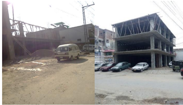
Figure 22. (Left) and (Right): A commercial plaza being raised during the course of documentation on main road, Samanabad
