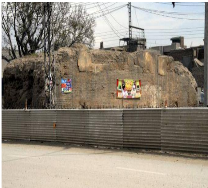
Figure 9. Dilapidated hydraulic water tank system of Shalimar Garden
