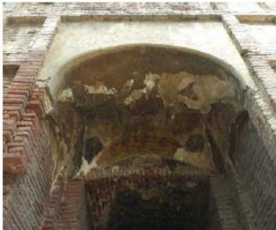
Figure 7. Nawankot Monument ornamentation decay
