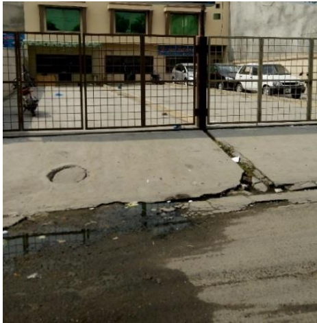
Figure 15. Effect of commercialization on roads and pavements
