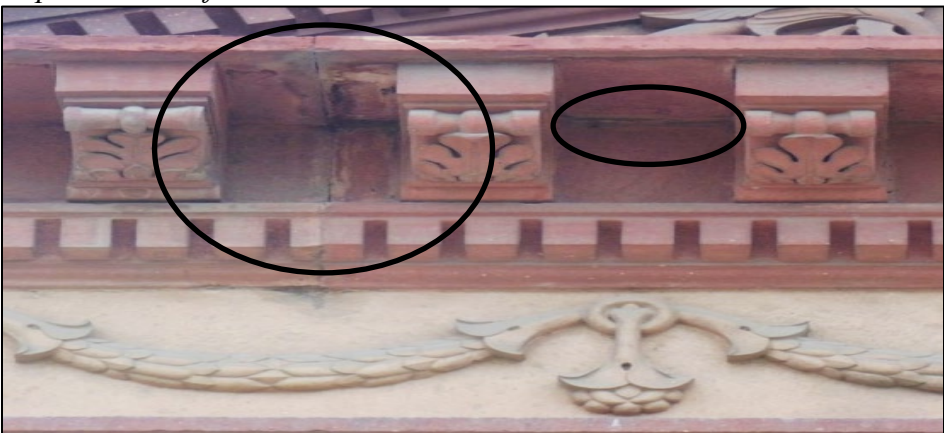
Gaps in Joints of The Clock Tower
