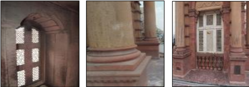
Black Deposits on the Exterior and Interior of the Clock Tower
