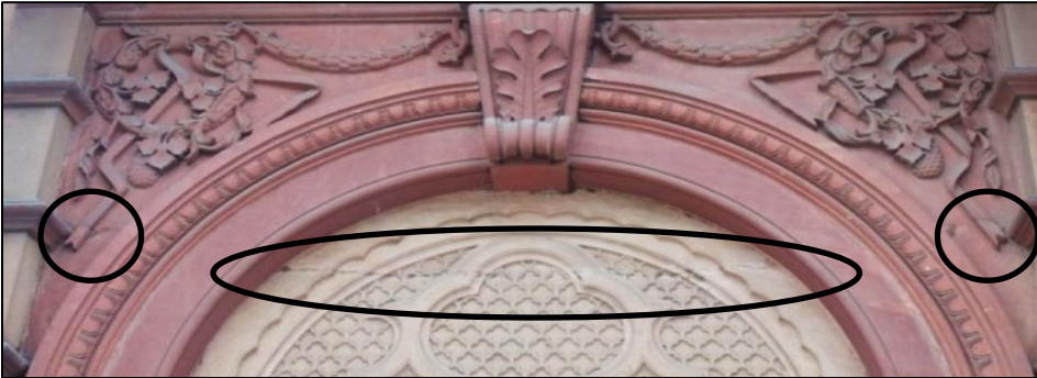
Cracking on the Ground Floor
