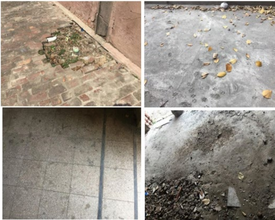
Floor Deterioration at Different Parts in the Haveli
