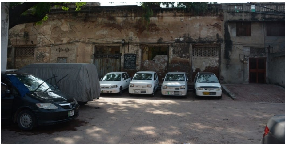
Courtyard of Haveli Dhayan Singh Showing Original Wall and Division of Haveli, Lohari Gate, Lahore
